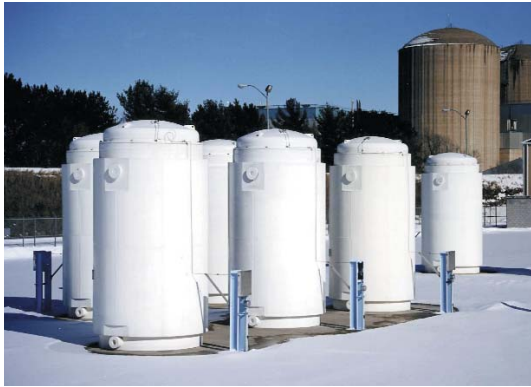
TN-40 Dry Storage Cask
